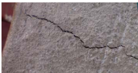
Fig. 8 Example of plastic shrinkage cracking
