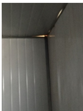
Fig. 5 Gaps between junctions [13]
