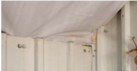
Fig. 14 Sharp edges in cladding [15]
