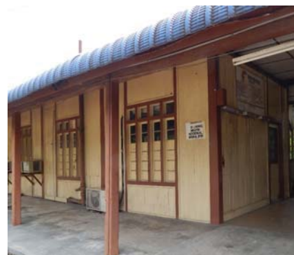
Fig. 21 The upper window part has been changed into glass to suit the usage of the air-conditioned
