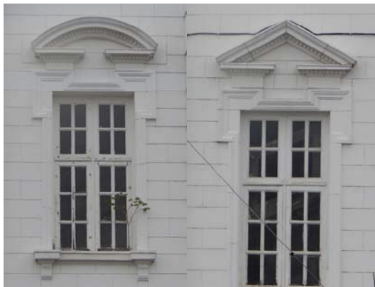
Fig. 23 (a) Circular and (b) triangular pediment as a window trims in Ipoh Railway Station
