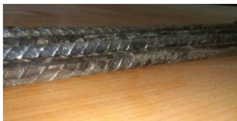
Fig. 4 Cleaned rebars after corrosion
