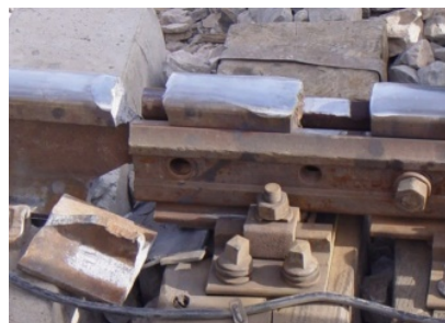
Fig. 1 Crack in rail bolt hole
