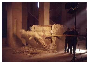
Fig. 5 Beirut National Museum. Rehabilitation after the civil war (1975-1991). Removing the cement box which covers a Roman Sarcophagus [4]
