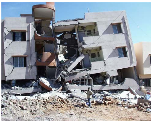
Fig. 1. Example of a horizontal layer with survival space in the collapsed first floor. Photo: Michael Markus.
