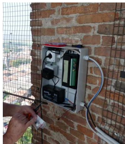
Fig. 4 E-log datalogger placed inside the bell tower of Lendinara
